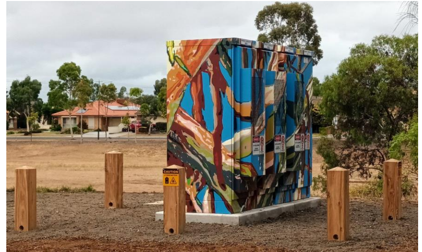
Powercor battery, Tarneit
