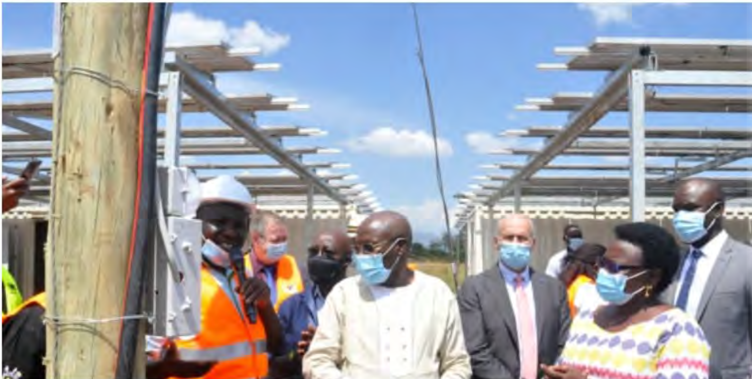
State minister for Energy Okaasai Sidronius Opolot (centre) flanked by the head of the European Union Delegation to Uganda, Mr Attilio Pacifici, during the commissioning of the solar-powered mini grid at Paloga Sub-county headquarters in Lamwo District on Tuesday. Photo/Tobbias Jolly Owiny
