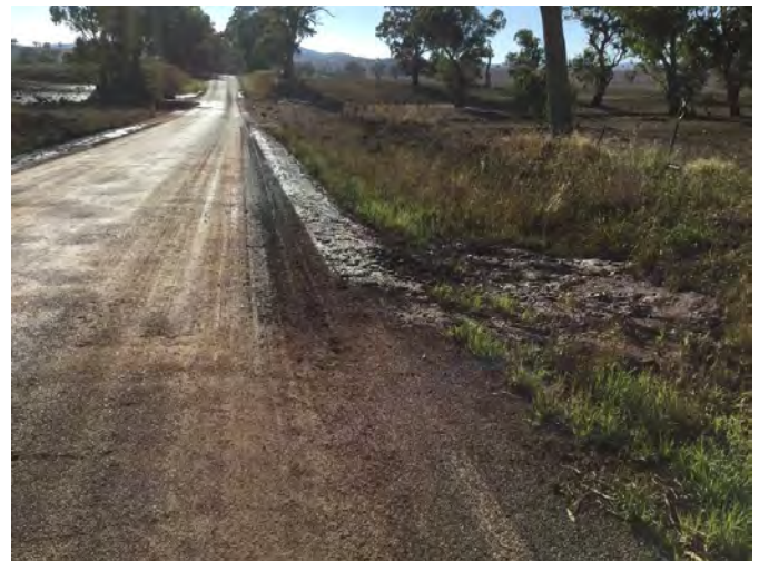
Cullinga Causeway in Cootamundra Shire requires an upgrade to reduce incidents of flooding
