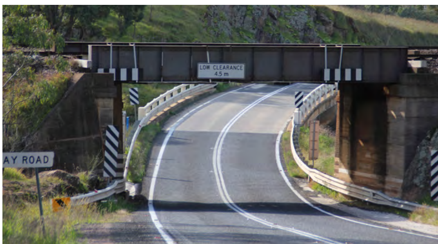
Suttons Lane is the high vehicle detour for the Gap Bridge (pictured) at Cootamundra
